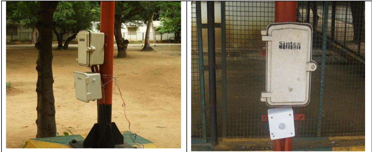
Automated street lamps (11 Nos.) are installed which saves 1425.6 units per year.
